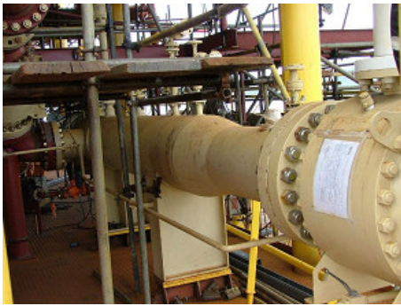
Installed horizontal pig chamber
