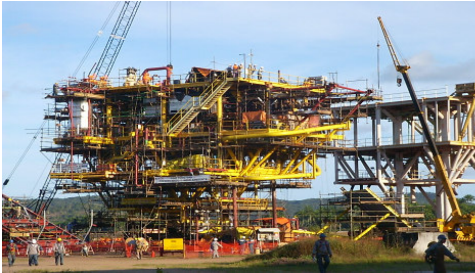
Set-up of platform by manufacturer. The vertical and horizontal pig chambers are marked.
